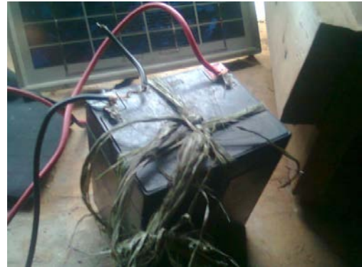
ig. 4.3: Panel Directly Connected to the Battery
