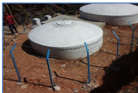
Rehabilitated water collection tank
