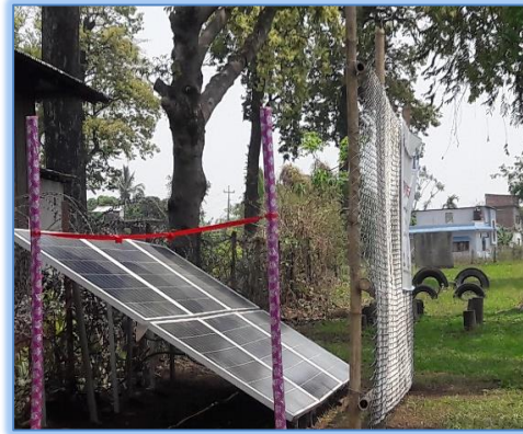
1.5 kWp Solar System in Snake Bite Treatment Centre at Letang, Morang
