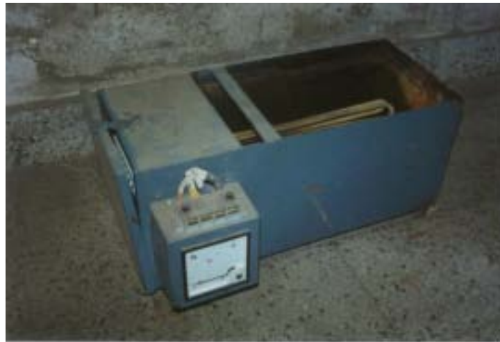
Photo A1: 18 kW Additional Dump Load with MCBs and Frequency Meter
