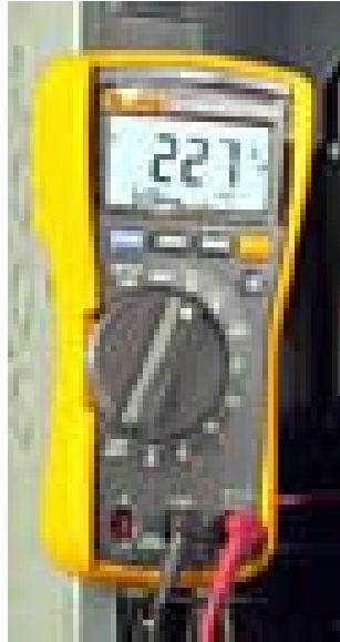
Photo A3 -1 –Digital Multimeter (DMM) used as Pressure Indicator
