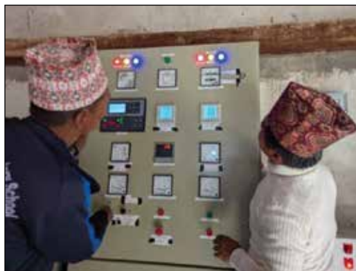
Figure 8: Control room of the Jhumsa Khola III Grid Interconnected Micro Hydro Project
