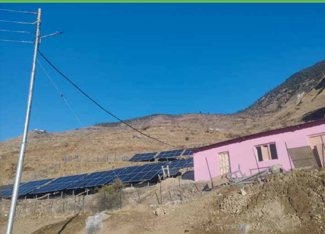
Solar Minigrid Project (120 kWp) installed at Soru Rural Municipality, Mugu
