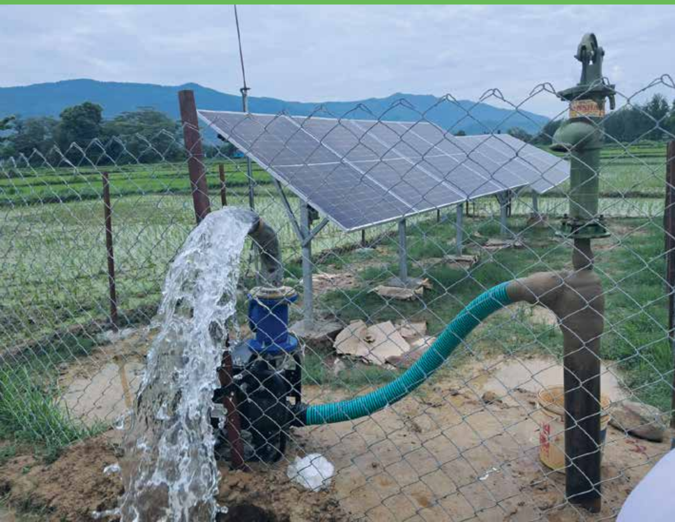
Solar Irrigation Pump at Susta Rural Municipality, Nawalparasi
