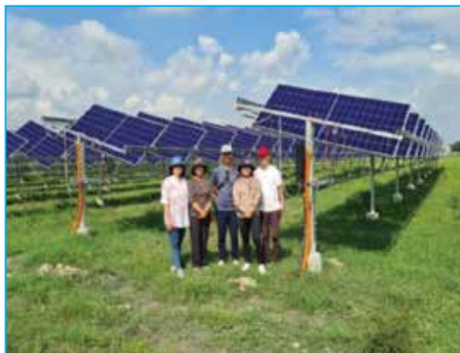
Grid connected Bifacial Solar PV System with 2-Axis Trackers installed at Hotel Mechi Crown, Jhapa
